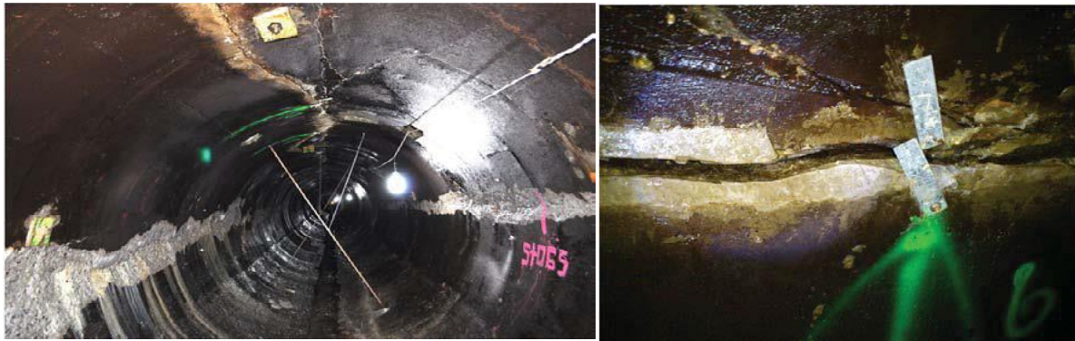
Figure 2. Stretch of damaged headrace tunnel and fracture detail [Source: Micheli et al., 2013]
