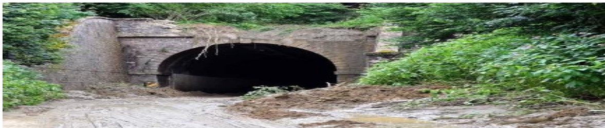
Figure 3. Landslide occurred at the Beaminster Tunnel [Source: Andrew, 2012]
